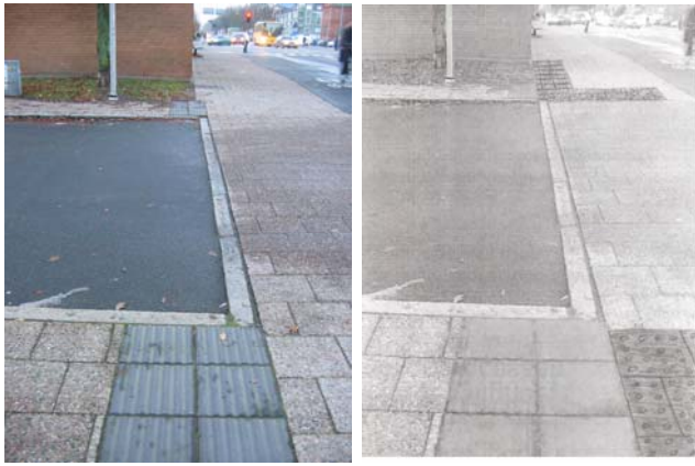
Picture 5 Suggestion for placing slabs with flat-topped domes as a warning at a raised pedestrian passage (right picture). Note that the sinus slabs have also been moved two rows laterally, according to the principle in Figure 3.
